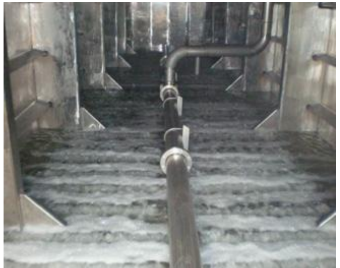
One of the CleanSea Aerated Basins shown during commissioning. In regular service this tank will contain ActiveCell Bio-Carriers and will be full of wastewater. The air will give the bugs the oxygen they need for respiration.
