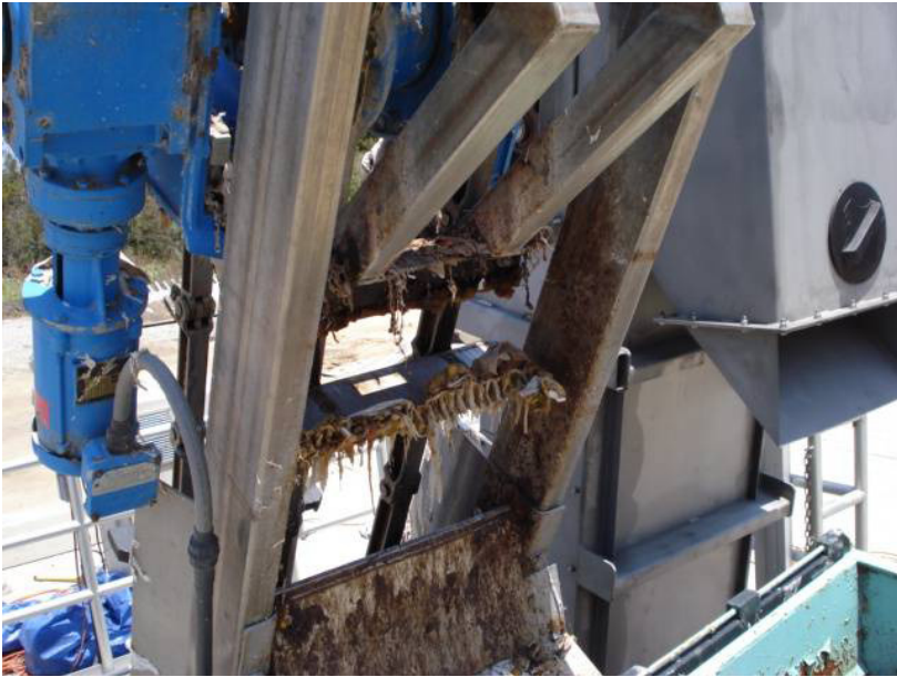
Debris collected on the old screen's chains and scraper mechanisms that frequently required cleaning.
